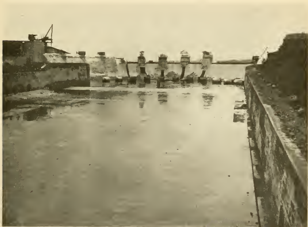
FIG. 3. GATUN SPILLWAY. MIDDLE SECTION STOPPED AT ELEV. 50. OPENINGS THROUGH DAM FOR CONTROL OF LAKE DURING CONSTRUCTION.
